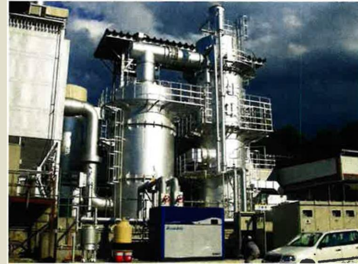
Compatible Modules - Gasification System
